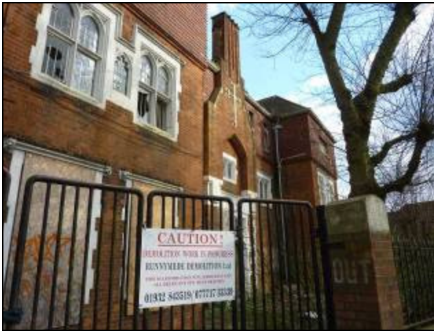
51 Drayton Green, boarded up and awaiting its fate
