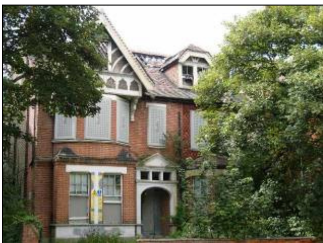
One of the once-fine houses on Hanger Lane subject to the latest proposals
