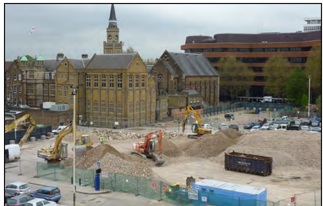
All that remains of the old Town Hall Annex
